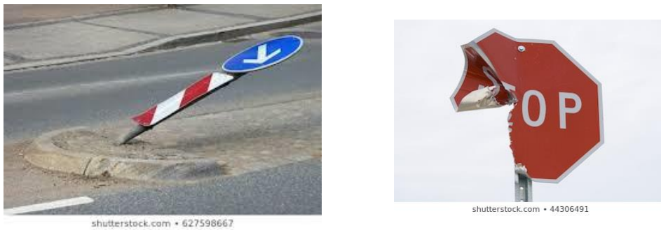
Figure 9: Examples of damaged road signs.
